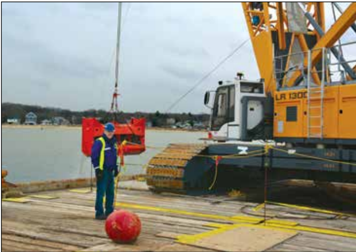
Jim Cleary on the deck of the dredge – a barge-mounted Liebherr crane using a 5.5-cubic-yard Cable Arm Environmental bucket.
