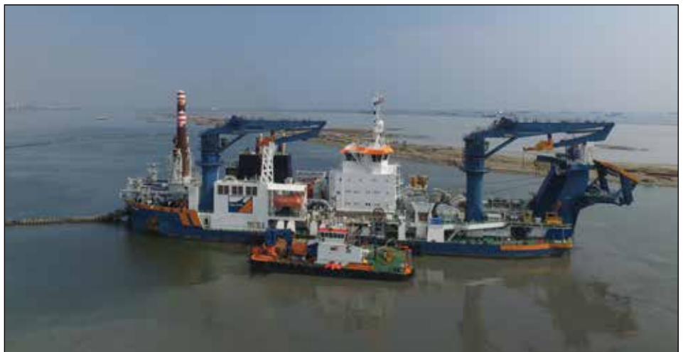
Self-propelled cutter suction dredge Athena will dredge an extra channel to the south of Marker Wadden.
