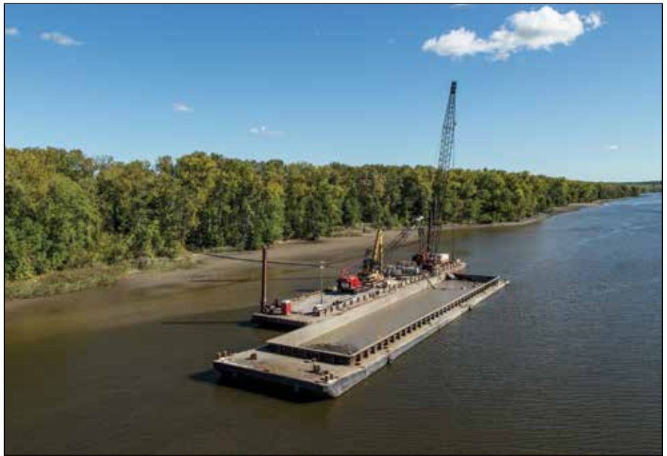
JT Cleary and Carver Construction performed maintenance work at Saugerties Harbor on Esopus Creek in upstate New York.
