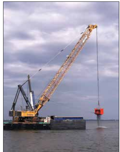
A JT Cleary dredge working on maintenance dredging of Fishing Creek at the United States Coast Guard Station, Annapolis, Maryland, with an environmental clamshell bucket.
